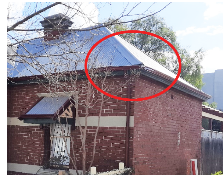
Photos: property damage at Aberdeen Street
